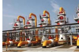
A compressor station [1].
