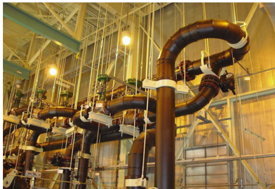
Figure 1.1: HDPE pipes with complex geometry butt welds in power plant [15].
