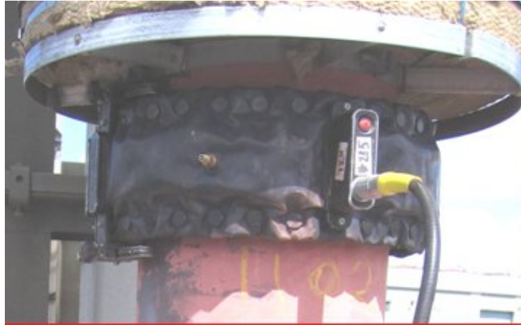
Figure 7.4: Picture of inflatable transducer ring used to perform guided wave inspections at Port of Liverpool power station.
