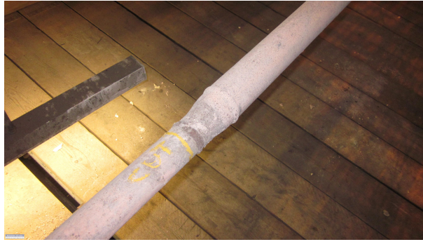
Figure 6.3: Photograph showing reducer connecting 2 inch supply to sootblower B29 with 2.5 inch main supply pipework
