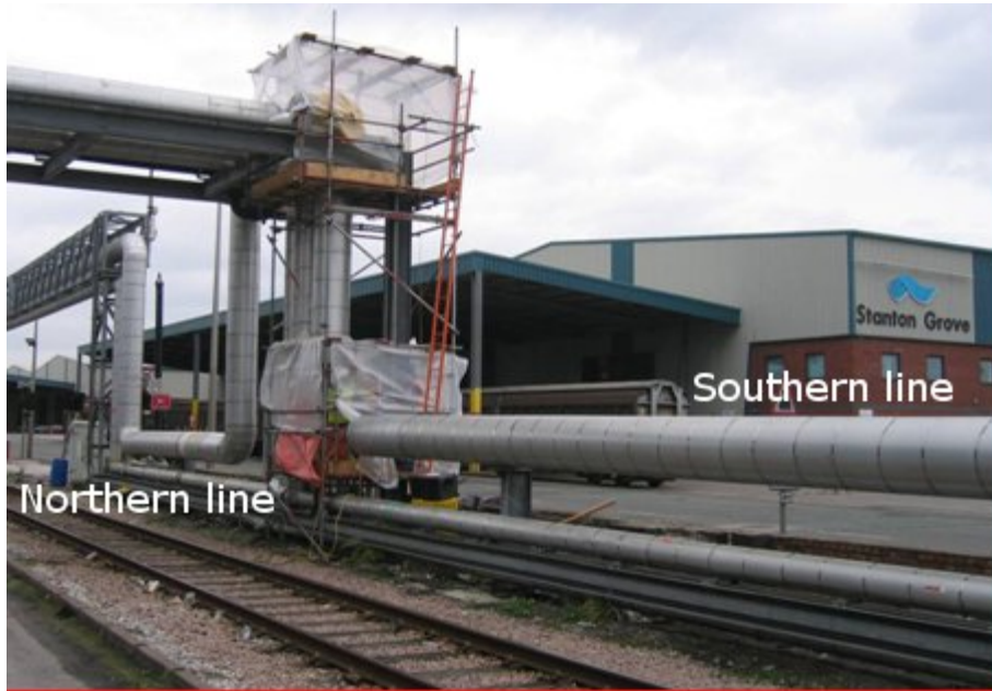
Figure 7.2: Picture of steam lines leaving Port of Liverpool power station with northern and southern lines labelled. A road crossing can be seen on the northern line.
