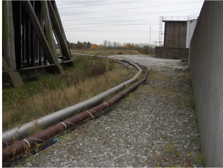
Figure 7.8: Picture of section of Fiddler’s Ferry BUFO oil line taking a curved path around a cooling tower.
