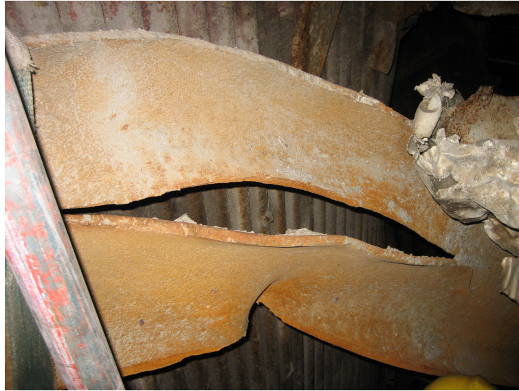
Figure 1.1: Picture of cold-formed bend after an axial crack resulted in the pipe rupturing.
