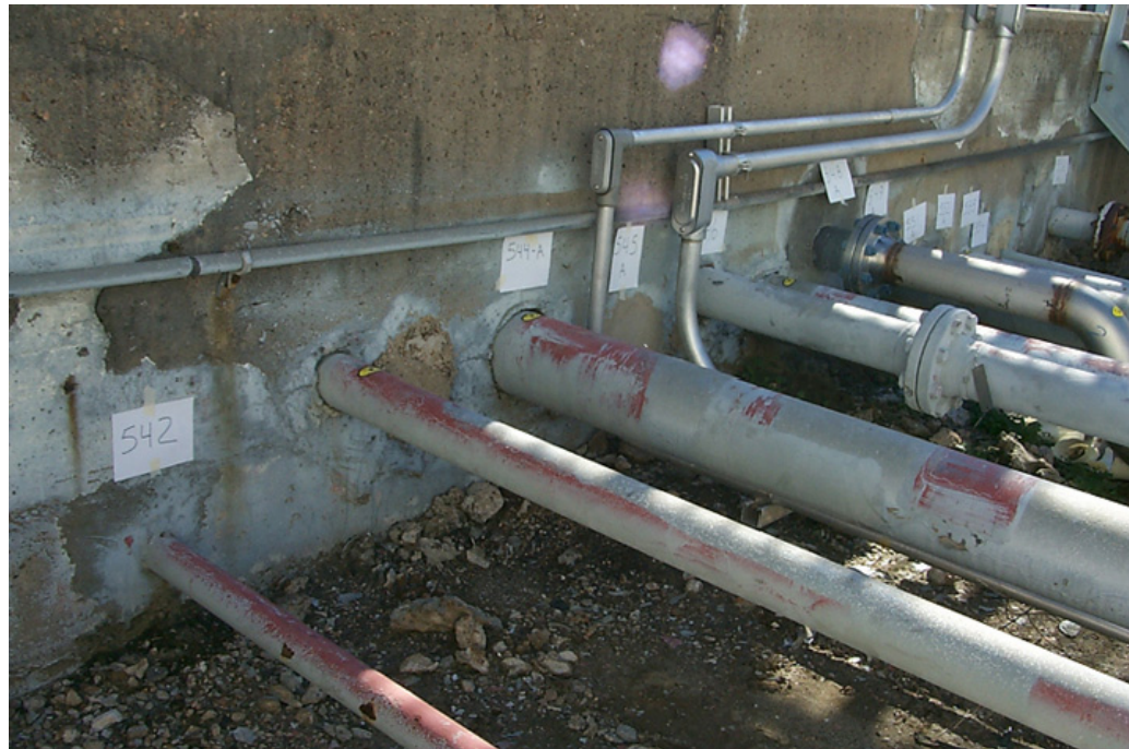
Figure 1.1 Example of applications where the areas of concern are not directly accessible: regions of pipelines embedded in concrete.
