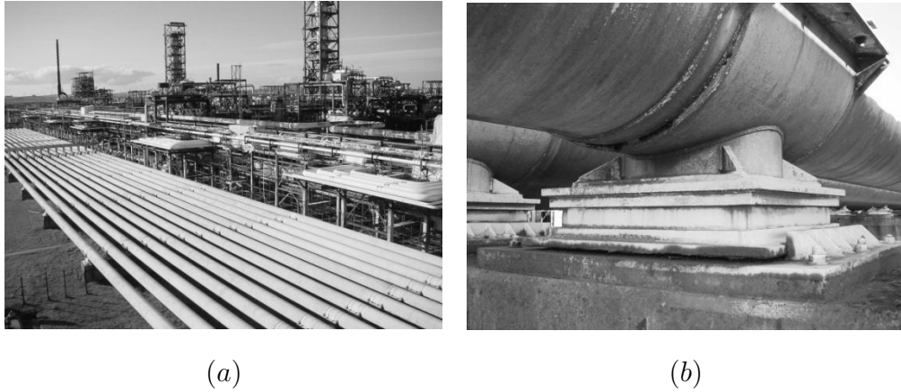
Figure 1.1: (a) slug catcher lines and (b) close up on a large pipe support. Photographs from Shell Global Solutions.
