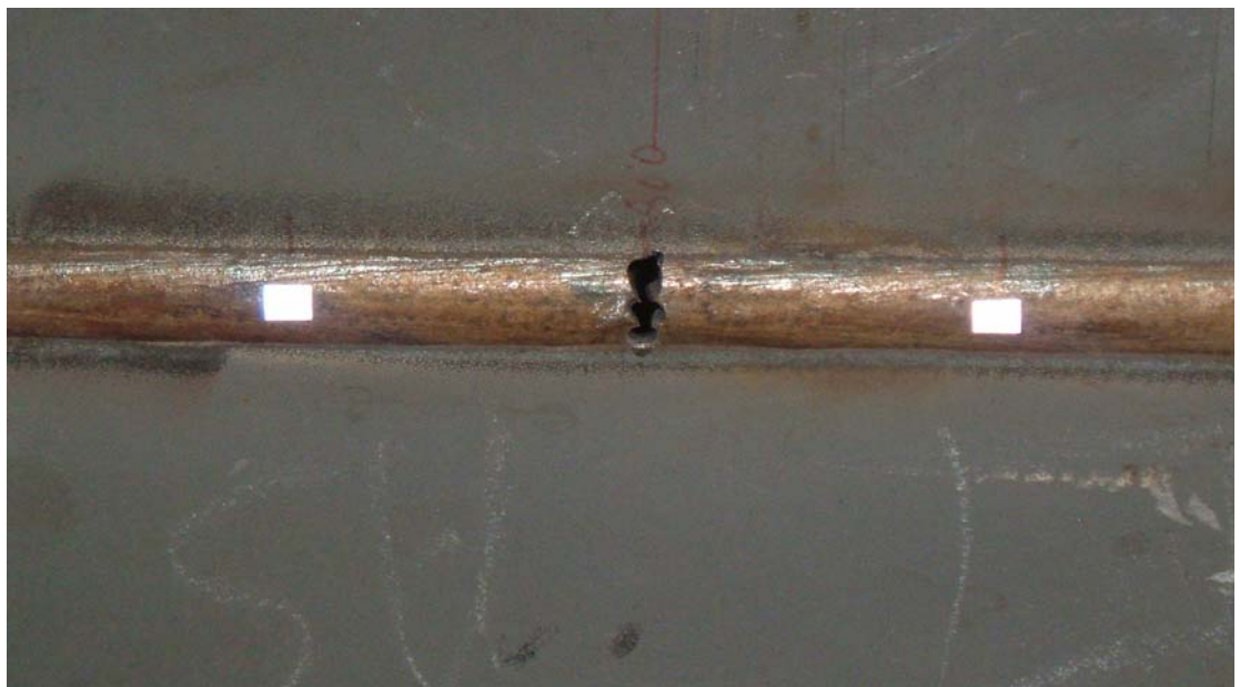
FIGURE 6.13: (a) schematic diagram of the model with a notch in the weld (b) Experimental plate with the notch in the weld
