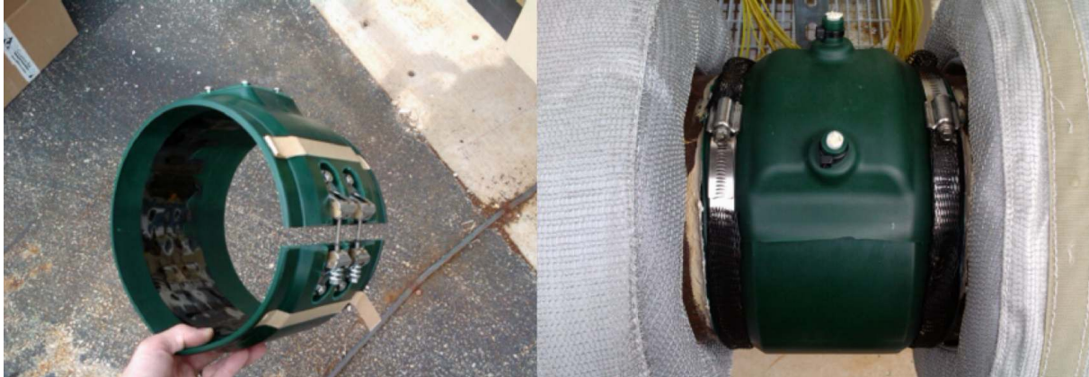
Figure 6.2: gPIMS® P1 sensor before and after its installation on the pipe loop.
