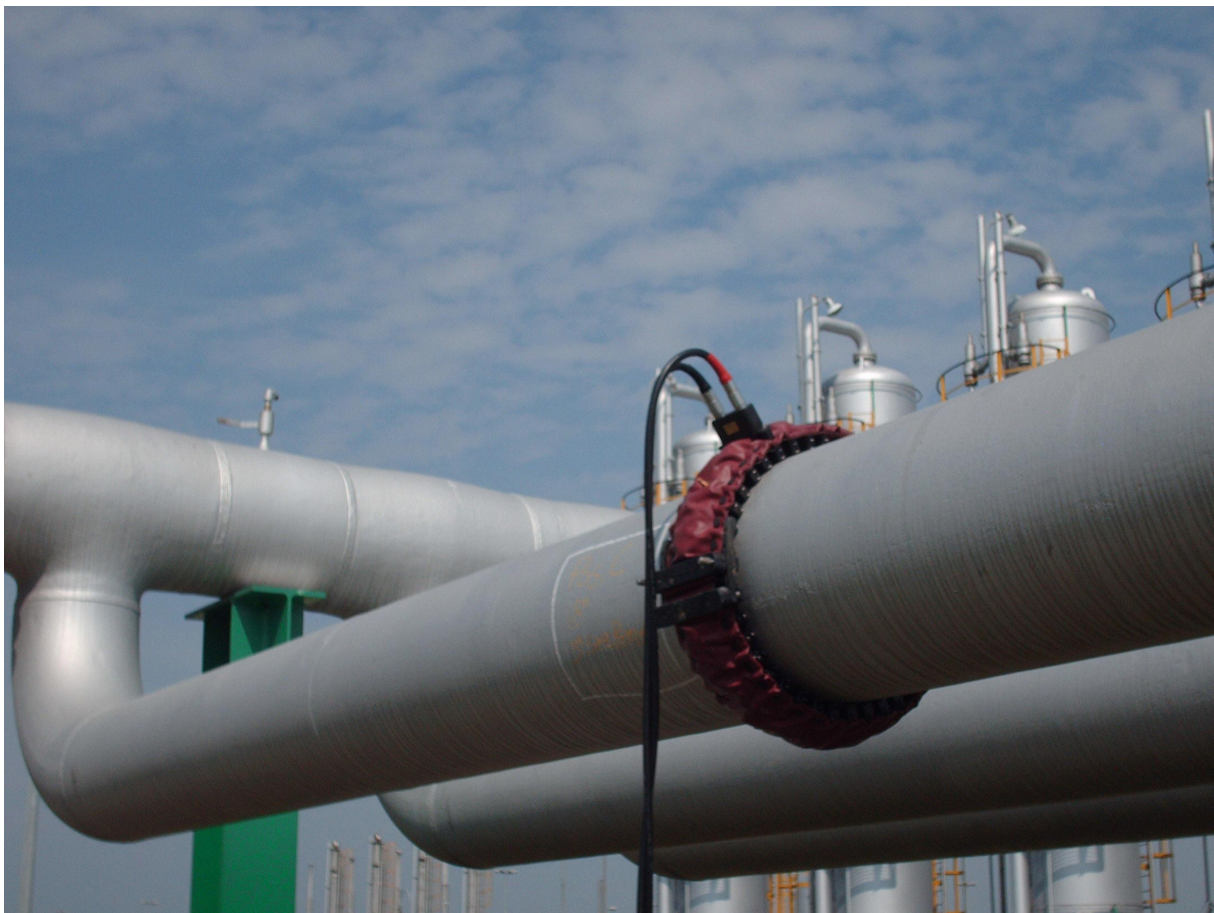
Figure 2.4: Typical example of a Guided Ultrasonics Ltd. flexible deployable ring sensor [54] installed on a pipeline and inflated during a guided wave inspection.
