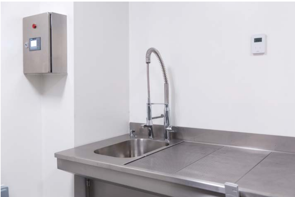
Top and middle: Surgical suites in the facility have been fitted with new state-of-the-art equipment, including a height adjustable perfusion table that can be used during the preparation of animals for surgery and in their recovery.
