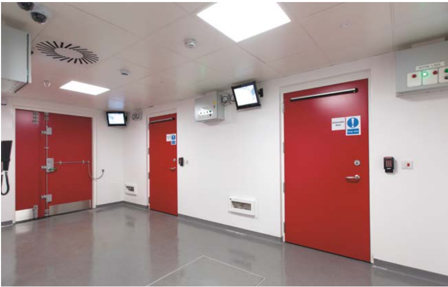
A new secure suite within the facility will be used for research of infectious diseases.
