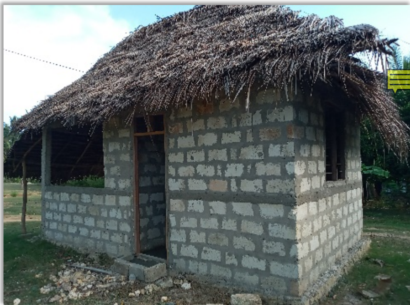
FIGURE 6: KITCHEN UNDER CONSTRUCTION (NEW KITCHEN WITH A FOOD STORE IN THE FINAL STAGE OF CONSTRUCTION AT MJINIKIUYU PRIMARY SCHOOL IN PEMBA)
