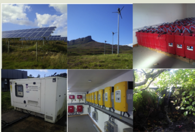
Components of the Eigg electricity system from top left: Solar PV arrays, wind turbines, battery bank, diesel generator, inverters system, hydropower turbine. Picture reproduced with permission from reference 96
