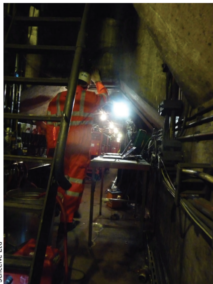
Cross-passages are congested!
