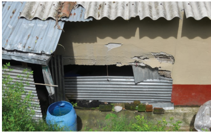
Wall destroyed by a landslide in Costa Rica
