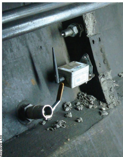
Wireless sensor deployed on a ring next to a grouting valve
