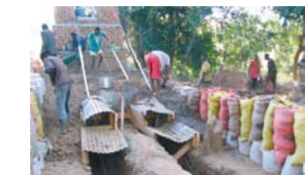
TOP: Building one of the towers. ABOVE: Retaining walls and shuttering for earth embankments leading up to the bridge. TOP RIGHT: A human chain passes bricks across the river.
