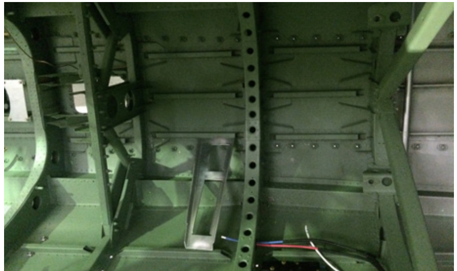
The fuselage and tailplane come to Biggin Hill from Airframe Assemblies on the Isle of Wight, having already received the camouflage treatment from Vintage Fabrics, at Audley End. When they arrive, the fuselage and tailplane are just empty structures which require Paul Ager’s team to fit systems such as hydraulic, pneumatic, fuel, oil, coolant, instruments and flying controls. “We fit every item with the greatest attention to detail” says Paul, “using original drawings and photographs to make the aircraft operate and look as if it were straight off the production line. Once these systems are fitted it is then the turn of our electrician to rewire the aircraft to the original Supermarine drawings.”
