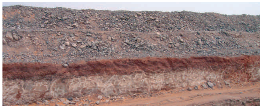
Figure 3 - A continuous, 1.5m band of grey-white dolomitic hardpan, with a strength higher than concrete, underlying a thin layer of reddish brown loose sand and gravel
