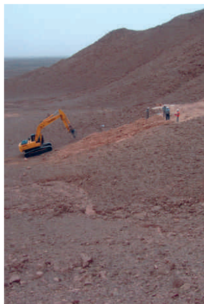
Figure 4 - Trial pitting at the base of a major cliff line that the proposed pipeline will have to ascend
