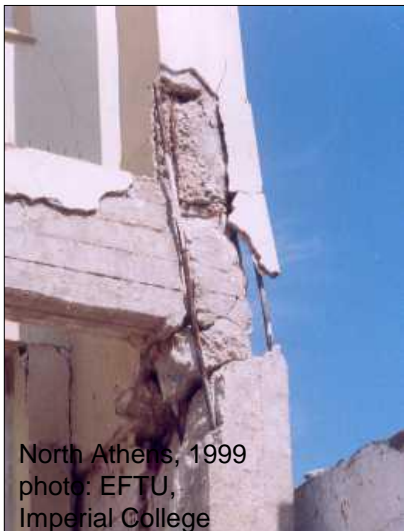
Inadequate detailing at critical zones
