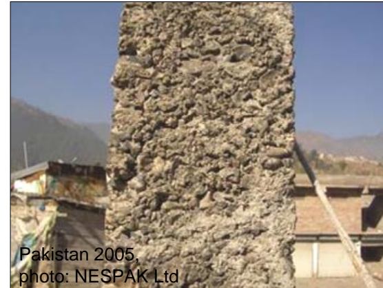
Use of poor quality concrete
