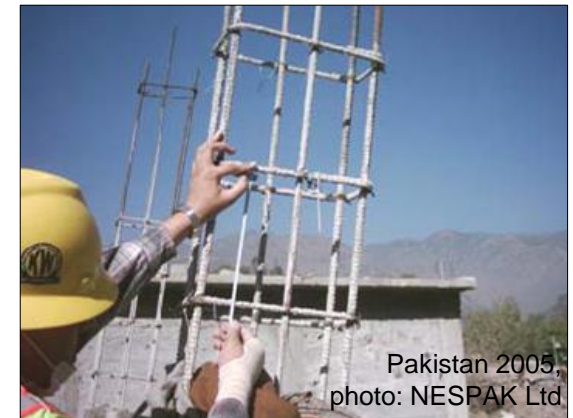
Lack of design/supervision
