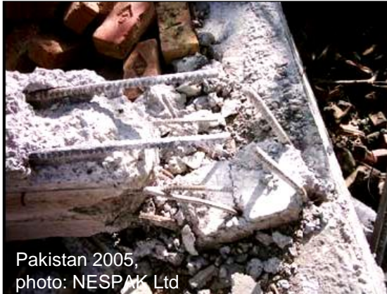
Poor anchorage & lack of confinement
