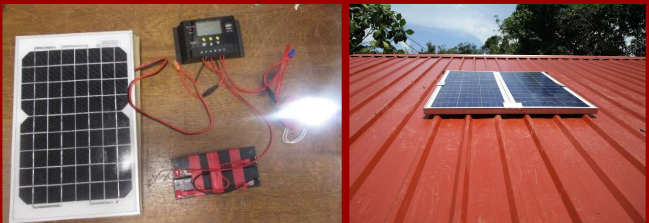
Figure 2: Prototype of the off-grid solar panel system (L) and the as-built system in Kampung Palipikan, Sabah, Malaysian Borneo (R).
