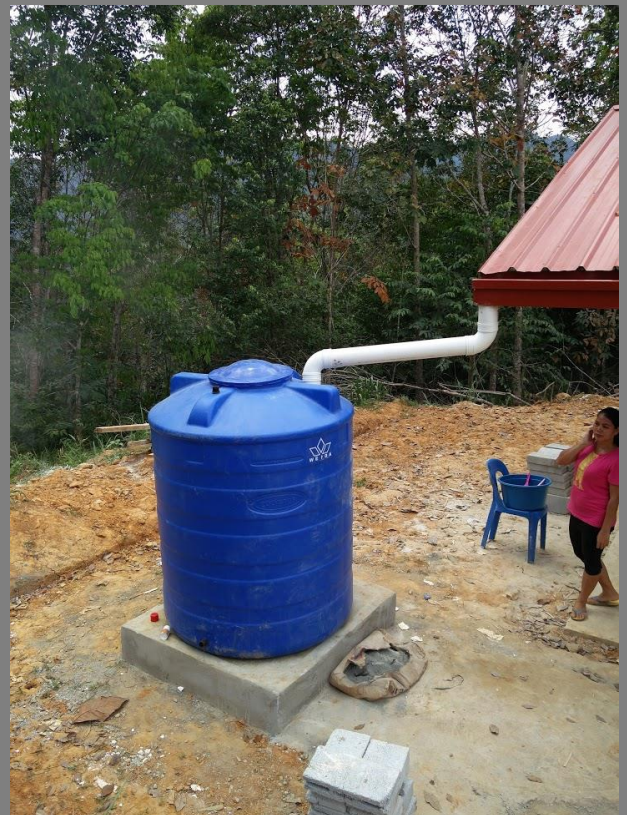
Figure 41: Rainwater Harvesting System
