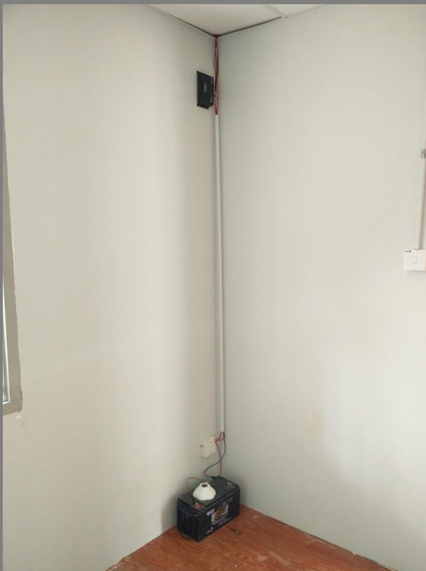
Figure 40: Wiring connecting to the charge controller and battery.
