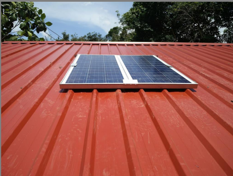
Figure 35: Solar panels attached onto the roof.
