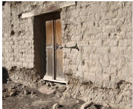
Erosion of base of wall
