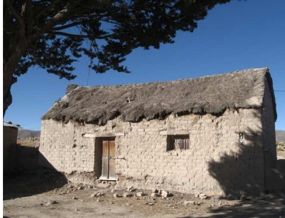
A typical adobe house in need of repair
