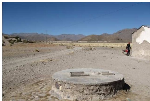
Well currently used by the village. Note uncovered openings.
