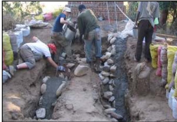
Fig. 9 – Setting the cables in concrete. Boulders were placed down the sides of each trench to reduce the volume of concrete required.
