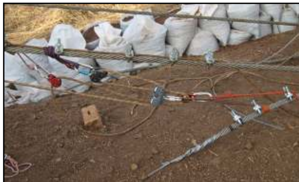
Fig. 4 – Three way pulley system used to tension the cables. An 11 mm static rope was used in the pulley system and attached to the 26 mm cable using grips. The end of the cable, which was tapered in order to feed it through the anchor block, can be seen in the foreground.
