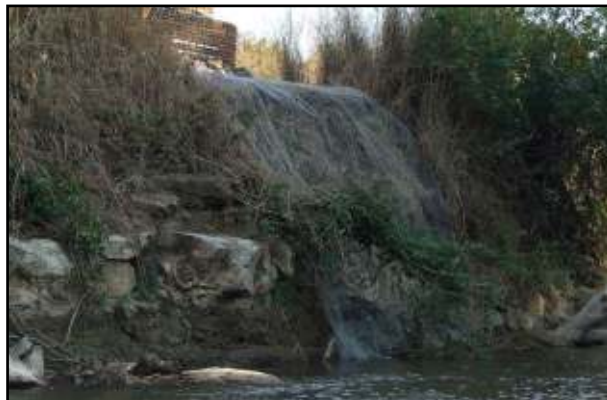
Fig. 12 – Wire mesh placed over the west bank to hold loose blocks in situ, thus protecting the bank from erosion.
