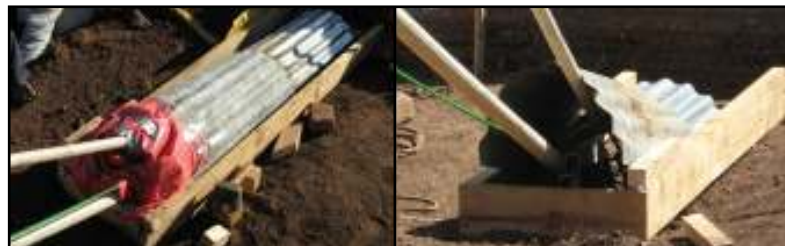
Fig. 8 – The shuttering placed around the cable trenches to keep earth out while building the embankment. Plastic pipes were also placed around the cables themselves to protect them.
