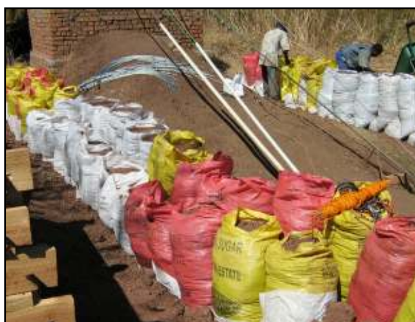
Fig. 6 – Construction of the retaining walls on either side of the west tower. Note the vertical offset in height between the front and back row of sacks in each wall.
