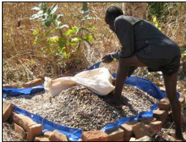
Fig. 5 – A worker empties his sack of aggregate onto the stockpile on site
