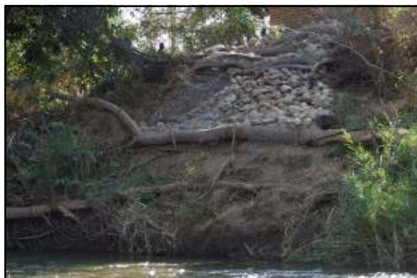
Fig. 10 – The eastern river bank protection. The idea came from natural protection offered by fallen trees and large roots behind which river deposits had accumulated. One such root naturally protecting the bank can be seen running across the lower bank in the foreground.
