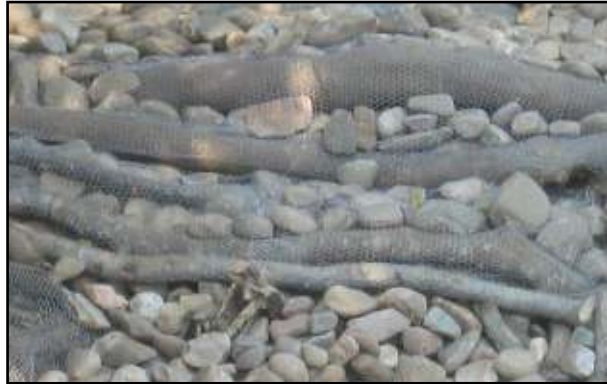
Fig. 11 – River bank protection on the east side. Logs were staked along the bank, rocks placed behind them and wire mesh used to cover them.
