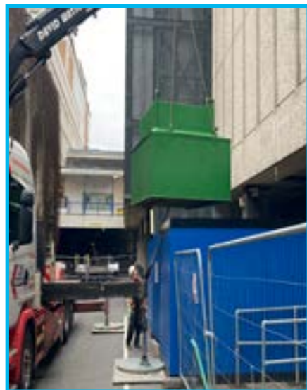
● TOP: HOARDINGS GRAPHICS, ROD COPPARD, ABOVE RIGHT: ONE OF THE TEMPORARY BOILERS, ABOVE: AN OIL TANK IS CRANED INTO POSITION
