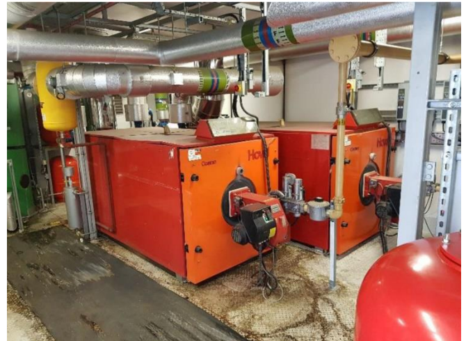
Figure 6. Before: gas boiler - Bessemer roof
