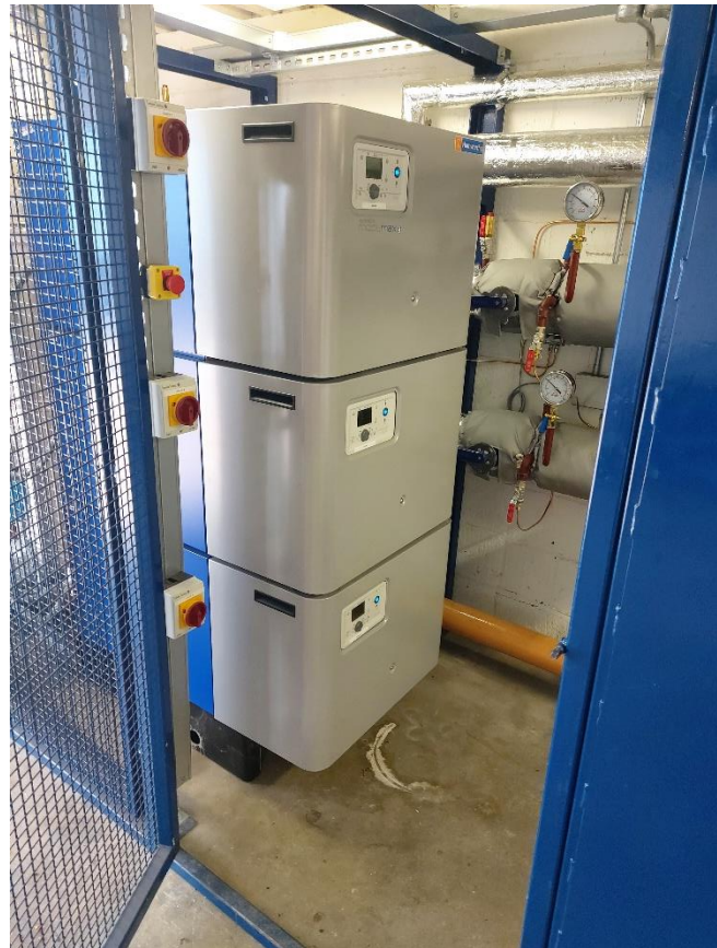
Figure 8. High efficiency Hamworthy gas boilers in 170 Queens Gate
