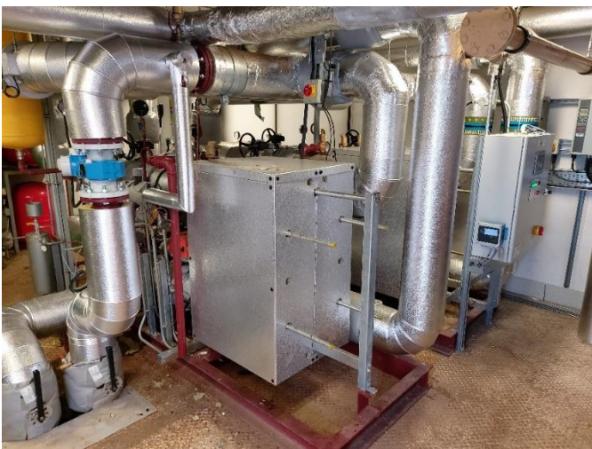
Figure 7. After: plate heat exchangers connecting Bessemer to the heat network
